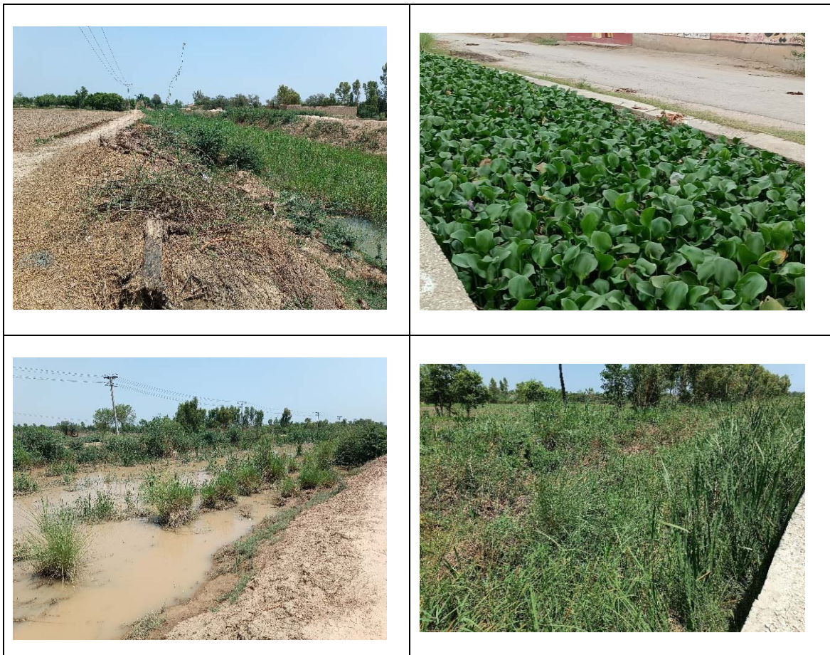
Figure 1.4: Heavy Silt, Vegetation and Sarkanda in Drains
